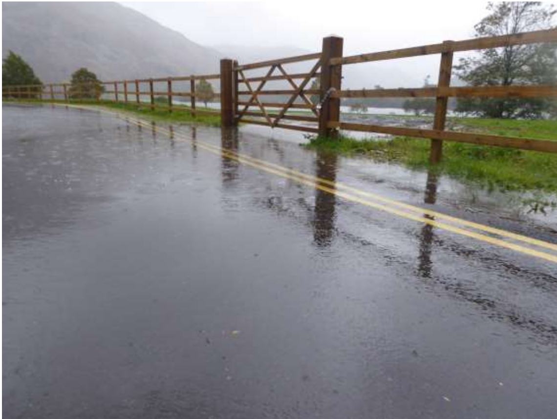
Water still pooling in the same place – once again suggest landscaping a run-off into Jenkins Field
