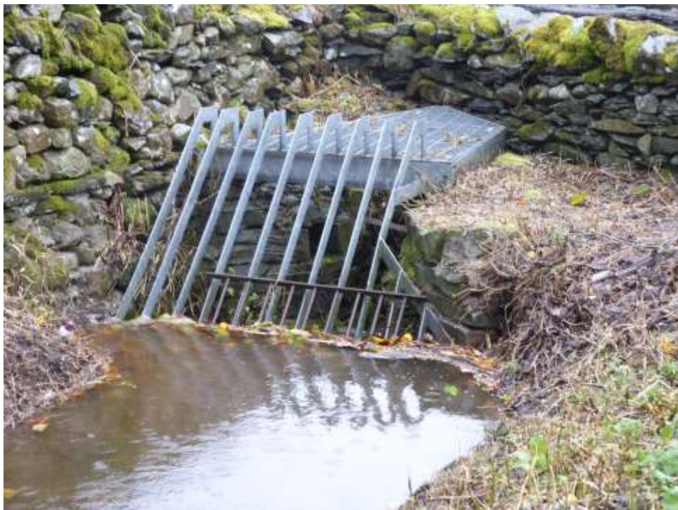
Grill needs clearing Carl!
